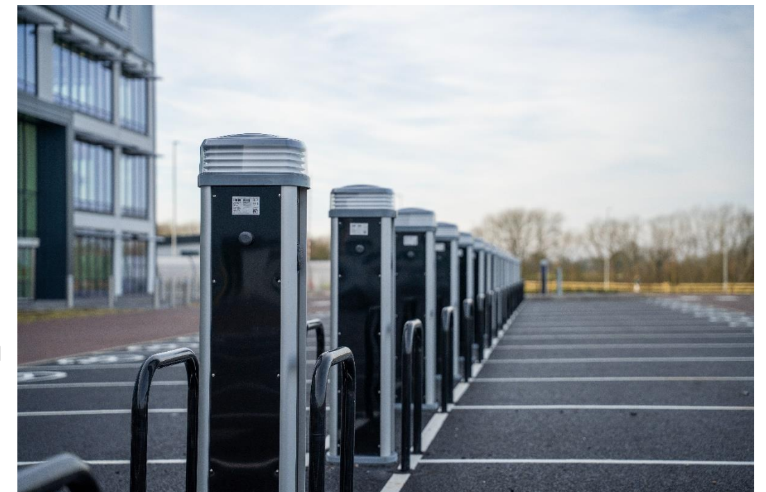
Fig 32. Examples of EV charging posts and bays within car park
