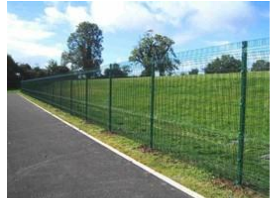
Fig 35. Typical Security Fencing
