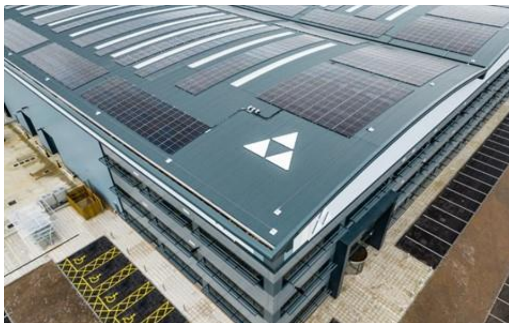
Fig 24. Illustrative example of a PV installation on the roof
